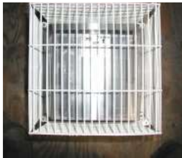
VIEW OF SAFETY CAGE
